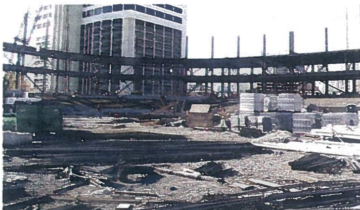
Construction materials scatter the site that would eventually take shape as Aces Ballpark. In late fall, the stadium's structure was already beginning to take shape.
