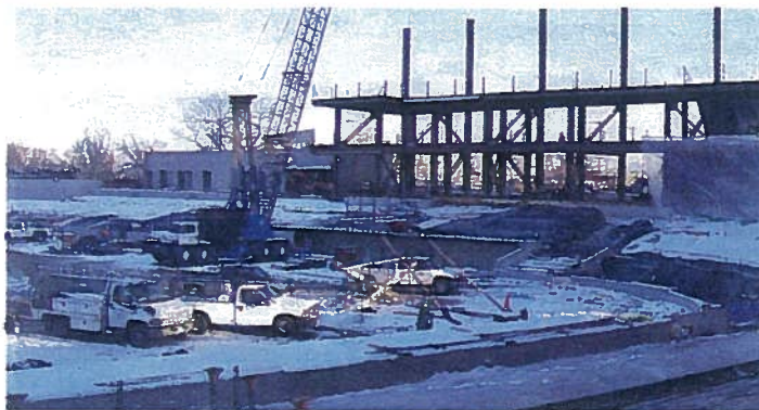
A December snowstorm frosts Aces Ballpark during construction. Despite the occasional inclement weather, Aces Ballpark was finished on time for its April 17 opening.
