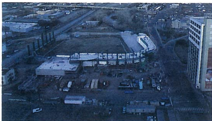
An overhead view of construction of Aces Ballpark. 275-300 construction workers toiled six days a week to get the stadium ready for the April 17 home opener.
