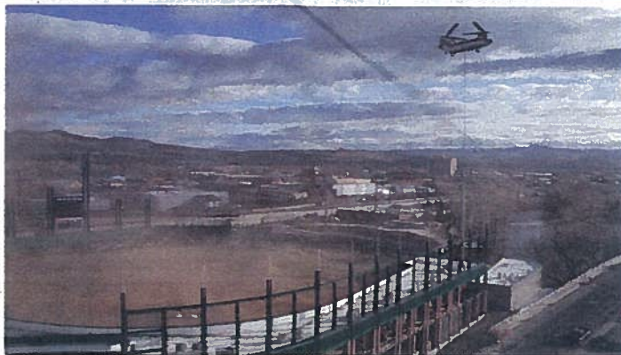
Light poles are flown into Aces Ballpark in March. The poles could not be constructed on site, so they were built on another property and transported by helicopter.
