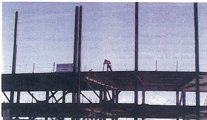
The last steel beams were set in place at Aces Ballpark by late November. Crews often worked six days a week to get the project done on time.
